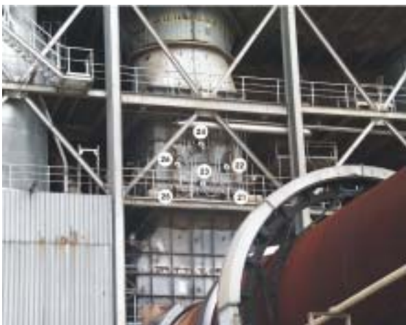
Fig. 1: SNCR process: Configuration of injection lances at a riser duct
